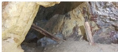
Figure 3. Underground workings present at the Prince of Wales Reef, Reedy Creek (CNW Group/Fosterville South Exploration Ltd.)
